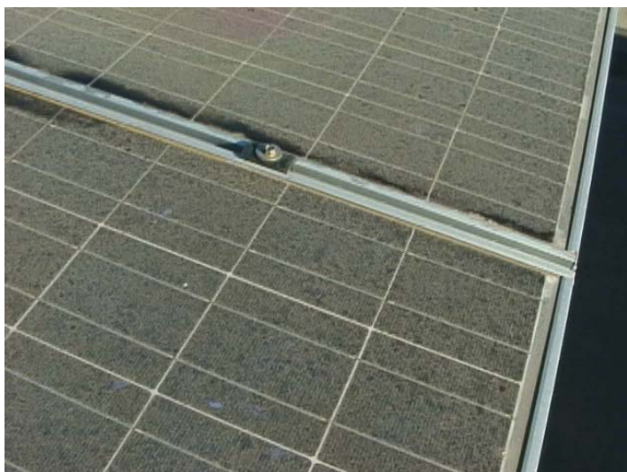
Fig. 1 An example of dust build-up on solar panels over time.
